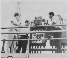
Tom Paddrick, Ben Kalis and Angel Rasmiñ checking a pump control panel.
